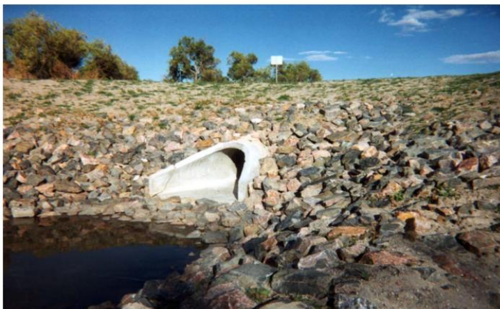
Photograph HS-13. Culvert outlets when left unprotected cause downstream erosion. The designer’s job is not complete until provisions are made to protect the outlet. Use of vegetated soil-riprap would blend this structure better into the natural landscape.
