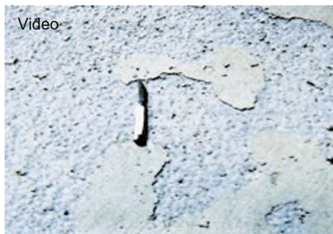
Fig. 3. Scaled concrete surface resulting from lack of air entrainment, use of deicers, and poor finishing and curing practices. (52742)
